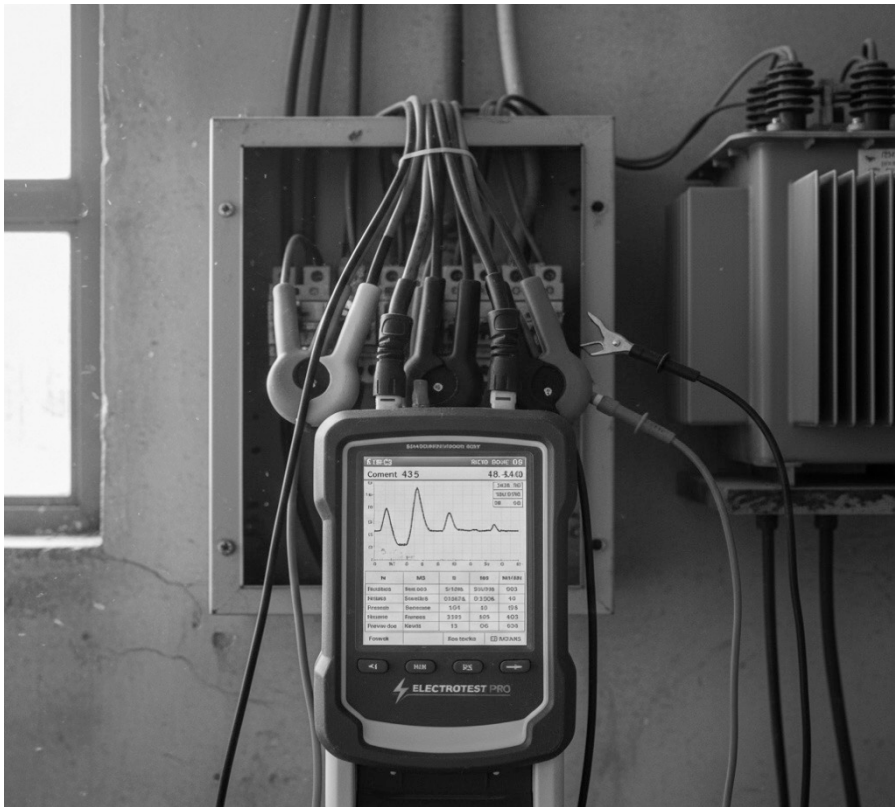
Fig. 7. A portable power quality analyzer, an instrument for field measurements on distribution networks.
